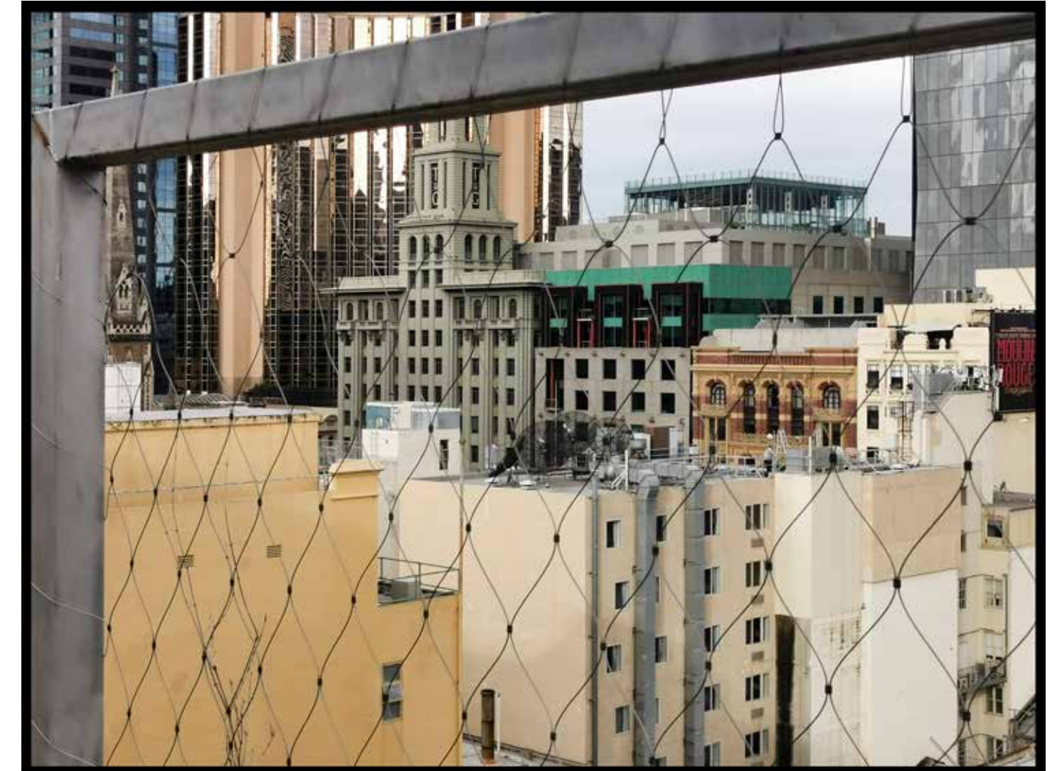
The supporting infrastructure to secure the screens to was already part of the designed structure
