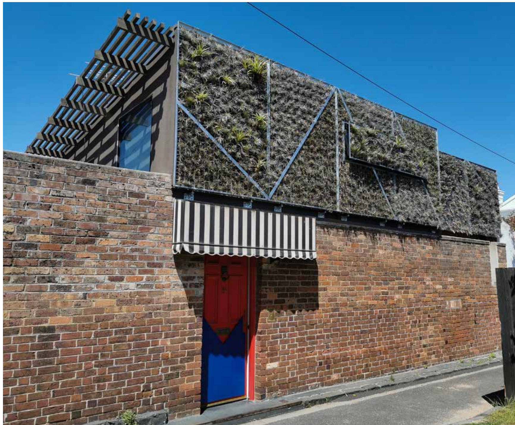
Second four panels of Tillandsia screens installed late October 2021. ( due to Covid lock down installation was dramatically delayed)
